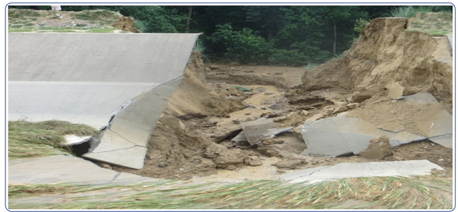
Figure 5: Embankment failure of Sikta irrigation project due to saltation in soil.(source: DOI)
